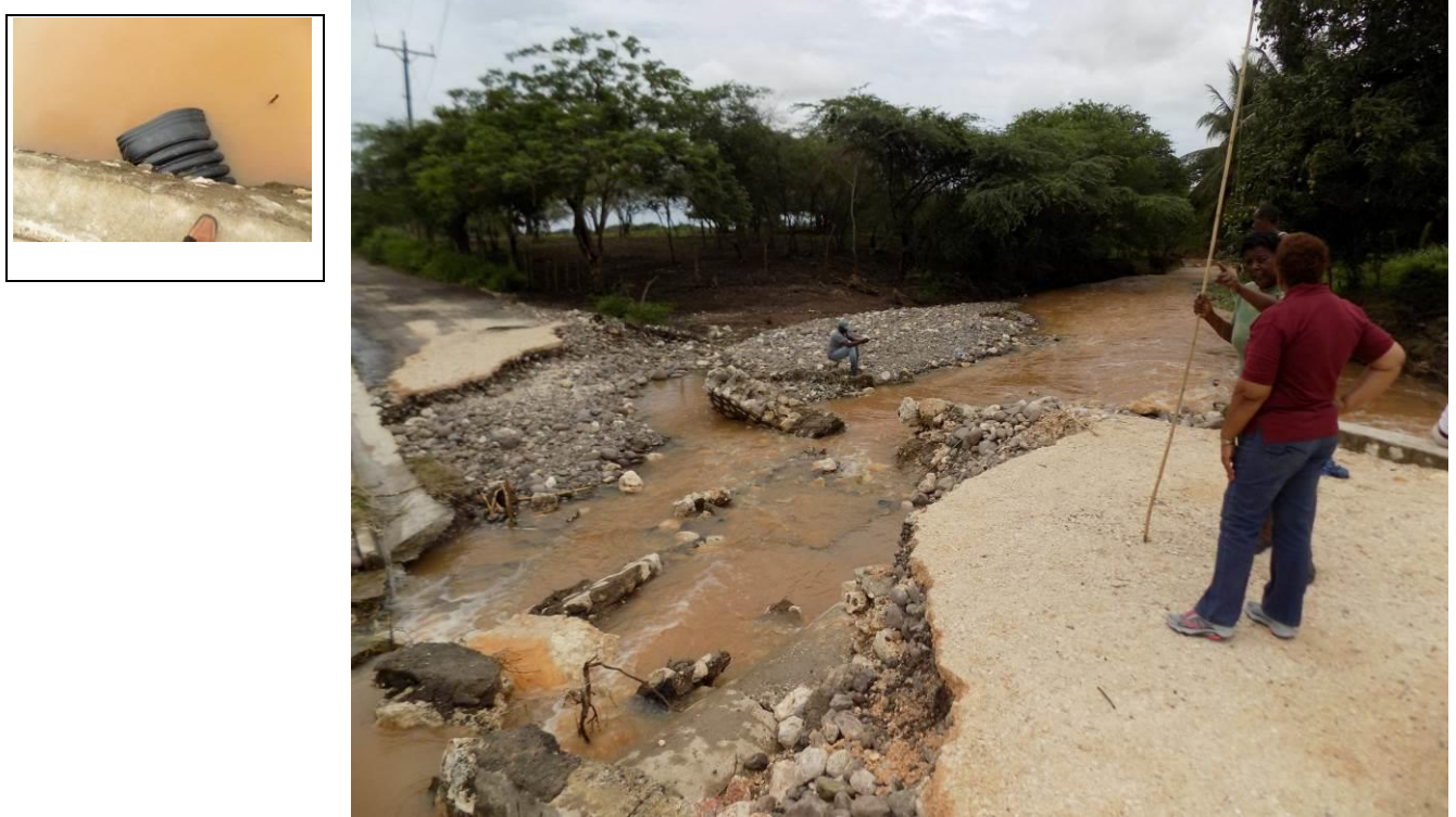
Figure 5.10: Washed out level crossing on a tributary of Rhymesbury Gully. Under-sized drainage (inset photo)
