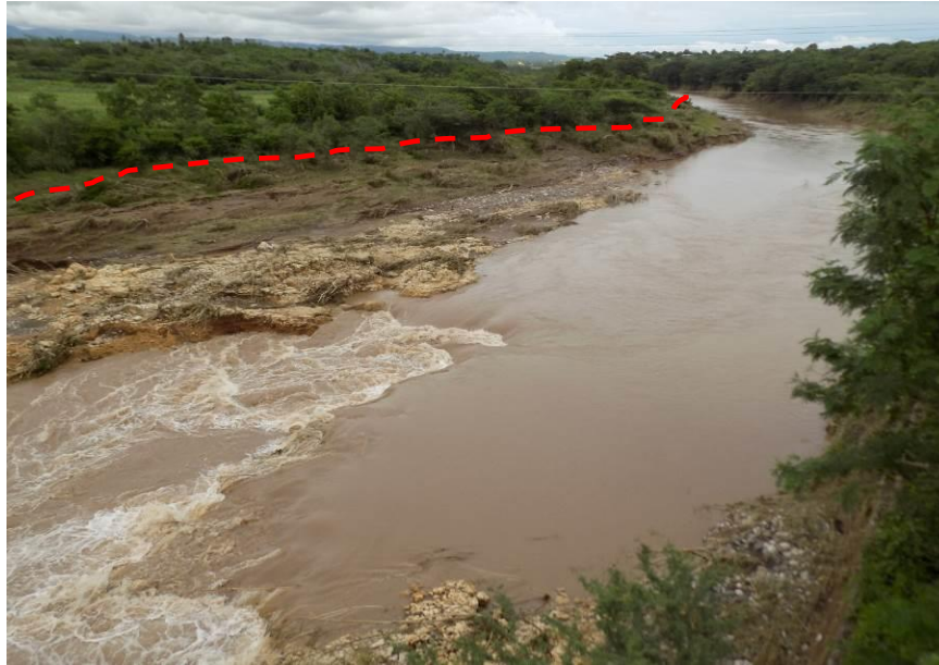
Figure 5.17: Upstream Rio Minho bridge. Note over bank flow and deep river bed scouring
