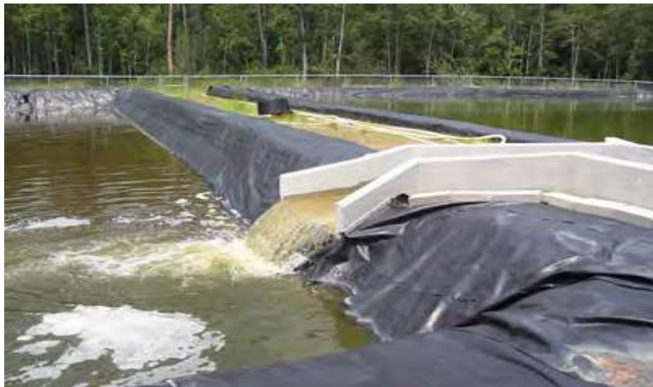
Plate 9.3 - Detention ponds used to reduce peak flows
